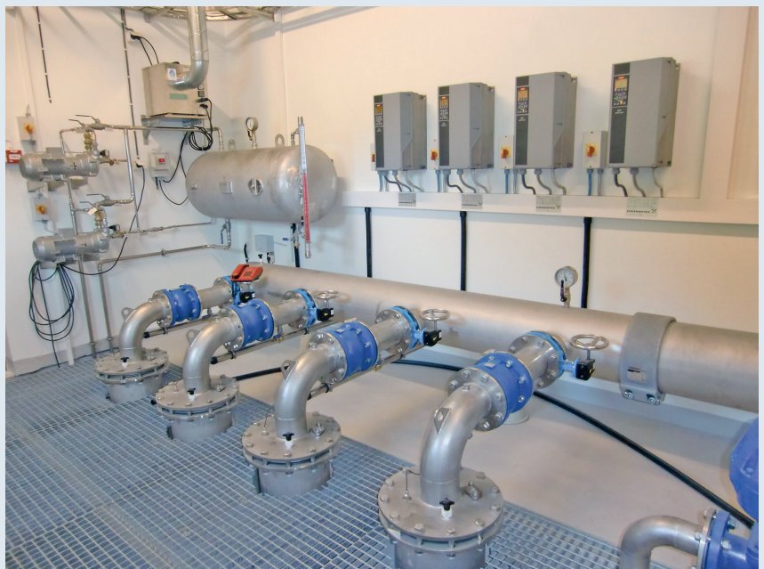
Figure 2: Raw water supply (Source: Hydro-Elektrik GmbH)
